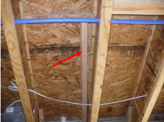
7) Two fireblocks should be installed along the rafter in the fireplace chase.
