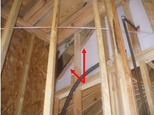
8) A Double TJI hanger should be installed on the floor joists above the rear door.
