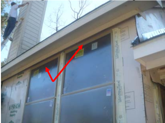
5) Thermo-ply and bitumen should be installed above the right elevation arch window.
